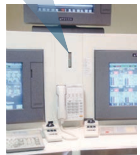
SIS Indicator in control room.
